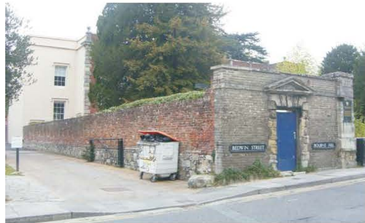
1. South-west corner of the Site with the west boundary wall, with glimpses of Council House and the dense planting of the East Garden behind, detractors include weeds along base of the south wall and location of the litter bin
